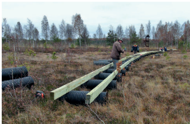
Plastikiniai vamzdžiai panaudoti tako pagrindui Plastic pipes were used as a basement for the path
